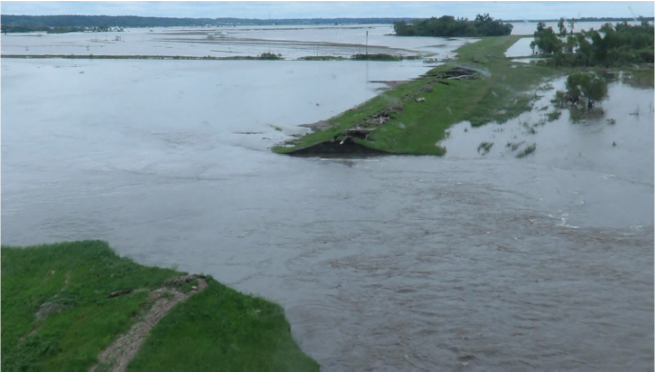
Helicopter view of L-536 damage following the March 2019 flood event.
