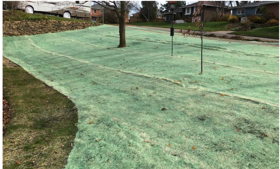
Erosion mats installed on slope after native seed was installed underneath. Young plants will grow through the mats.
